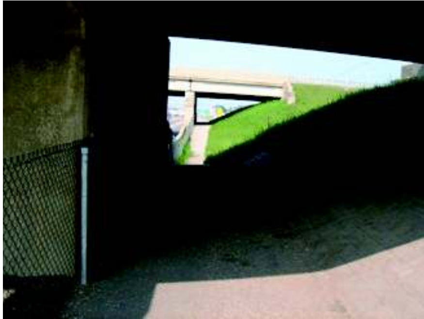
3. View looking west along the north side of West M-32 from under the northbound I-75 bridge.
